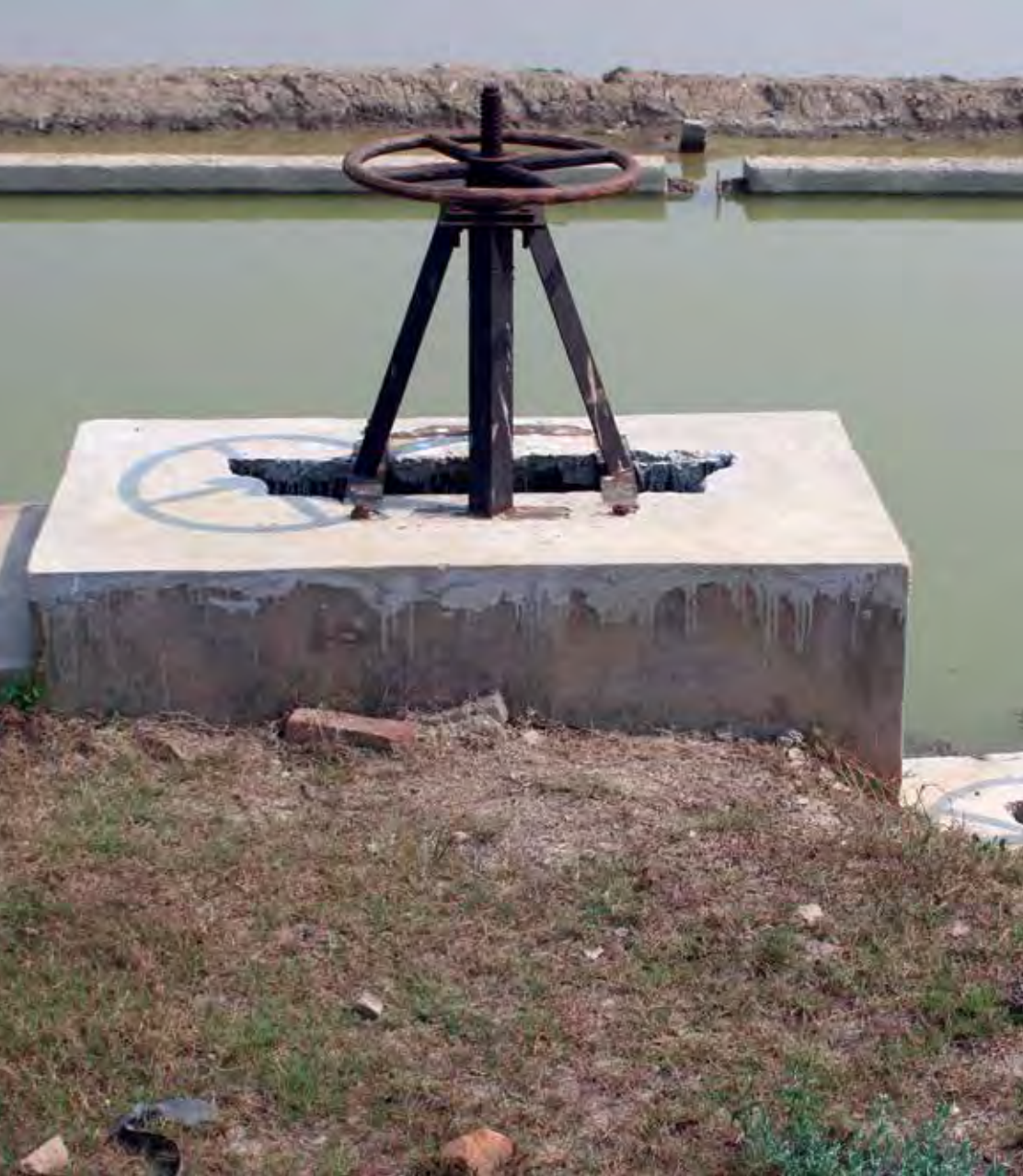
Reconstruction of three main feeder sluices at KRC of CIBA at Kakdwip
