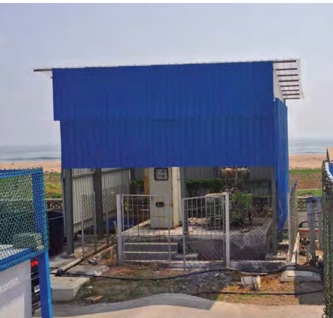
Renovation of Grill and shed around HT Electrical panel at MES of CIBA
